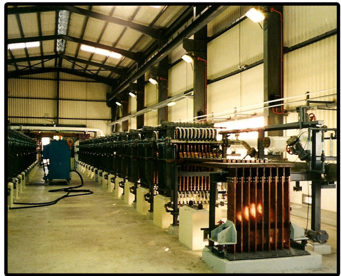
Chlorine Production Plant - 117 VDC 56kA Busbars
