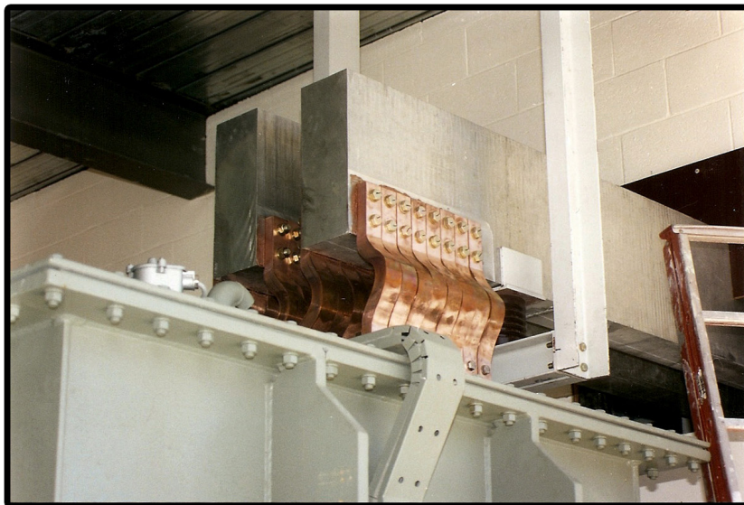
8MVA Transformer - Busbar AC Connection 400x 150mm Al
