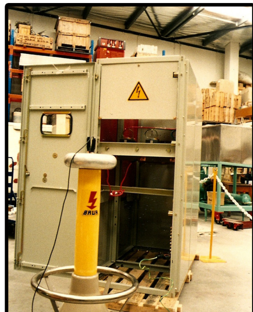
22kV > Switchboard QA Highpot Testing
