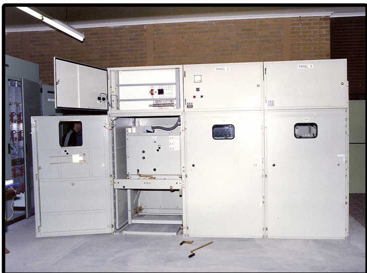
22kV Switchboard. Lilydale VIC Substation
